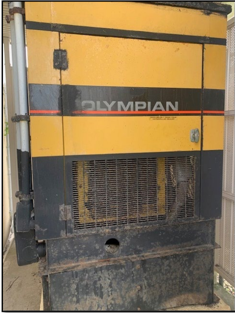
Exterior of Current Generator
